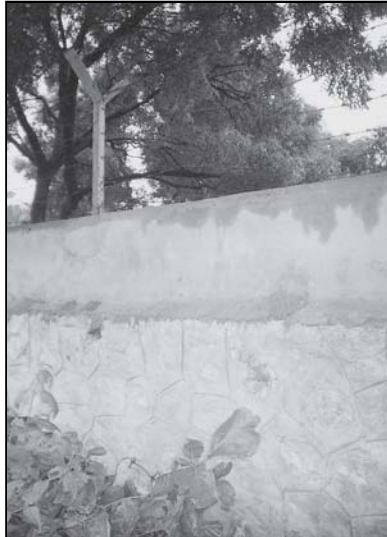
The boundary wall of the Coke factory raised to keep out protestors.
